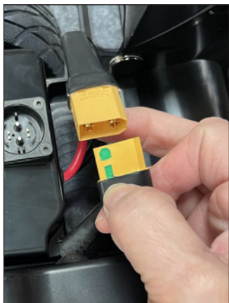
Figure N: Battery disconnected.
